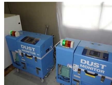
Figure 7 Continuous dust monitor on the premises
