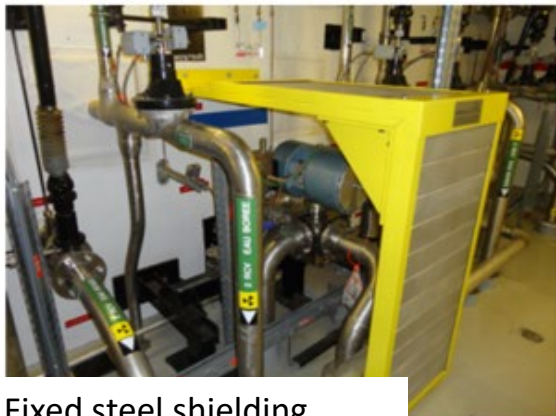
Fixed steel shielding
