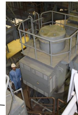
Condensate pump (in the case of Unit 2)
