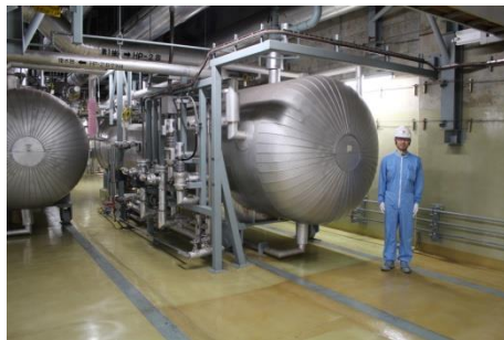
Feedwater heater (in the case of Unit 2)
