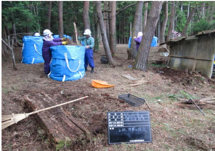
3) Packing work of the fallen leaves, etc. into the flexible container pack
