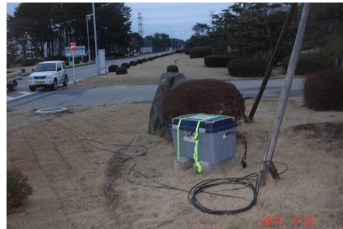
Portable monitoring post at main gate
