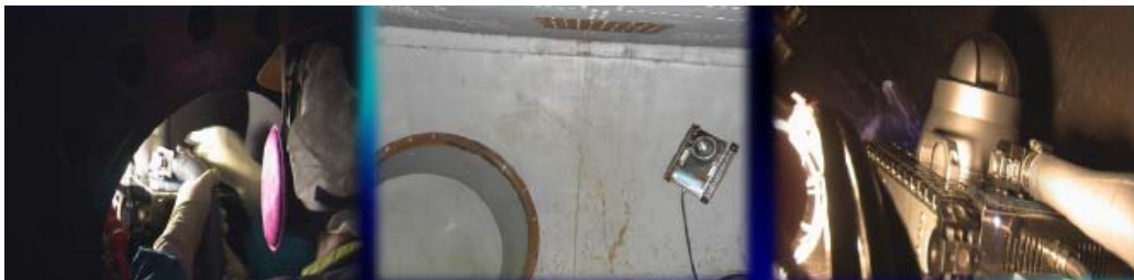
Steam Generator RMVS
